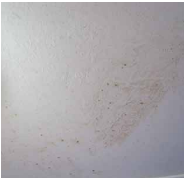
Figure 16 Bathrooms: mouldy ceilings
