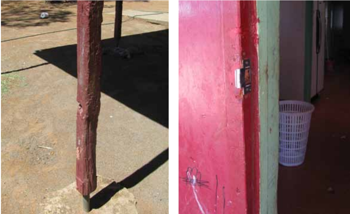
Figure 14 Poor quality of workmanship in Warlpiri Camp
