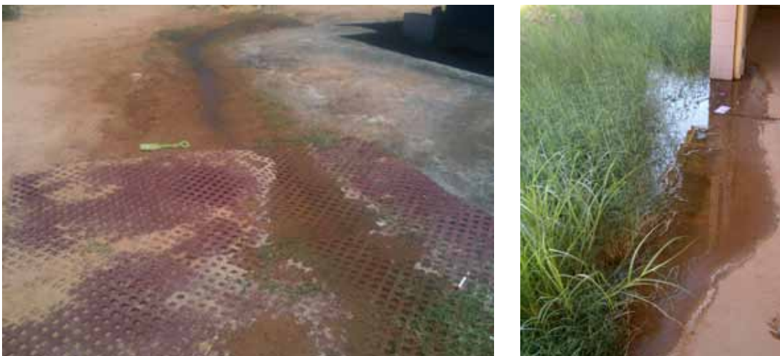
Figure 15 Water pooling in the yard
