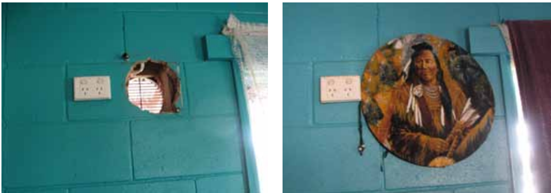
Figure 13 Incomplete work and tenant's response
