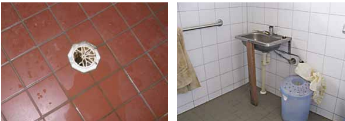
Figure 18 Bathroom floors: accessibility, workmanship and floor grates. Poorly fixed hand basin.
