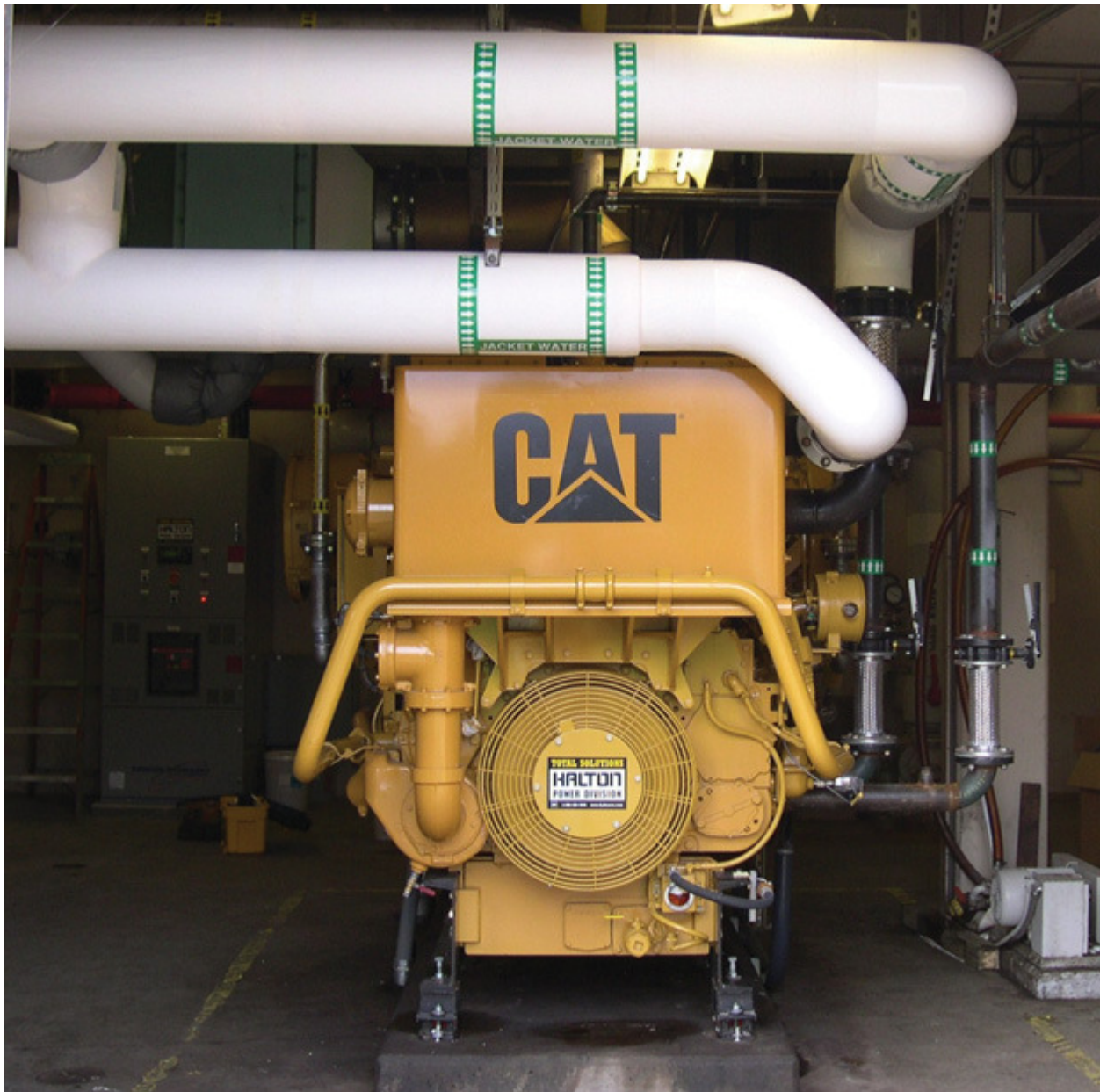
The engine-based CHP plant
