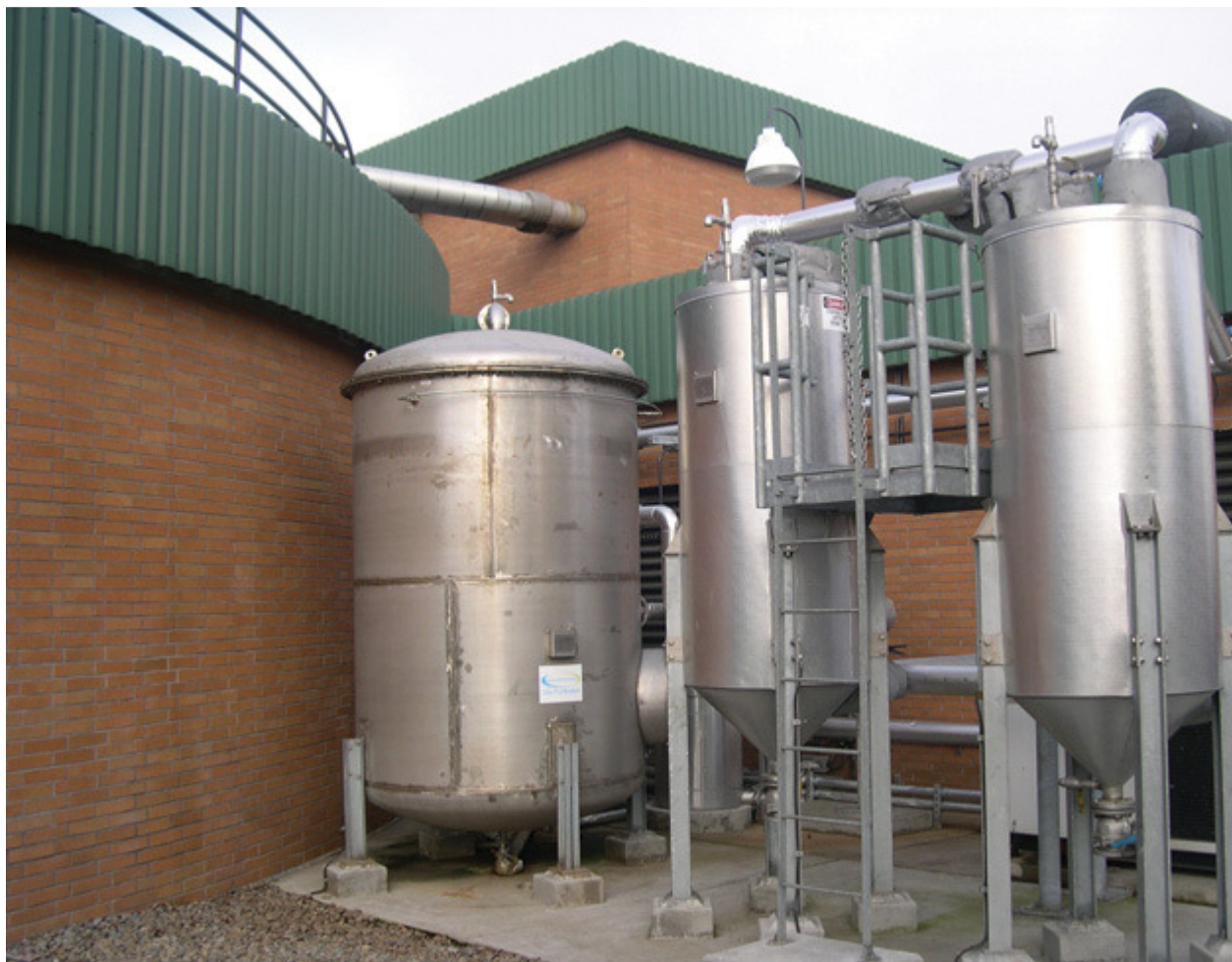
Gas treatment plant Source: City of Gresham
