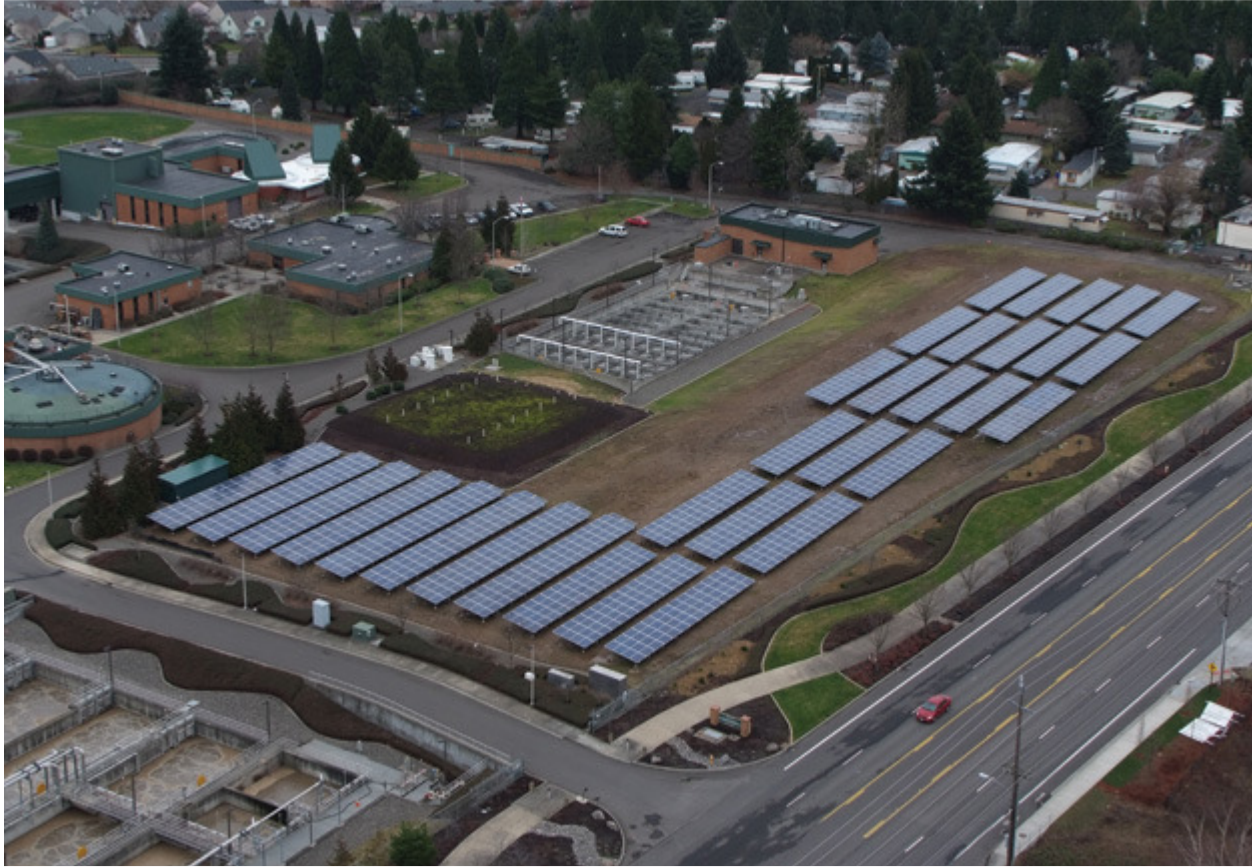
Aerial view of the solar PV installation Source: City of Gresham, SunEdison and REC Solar
