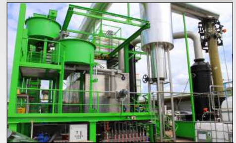
25 TPD Plant – Germany (2011)
