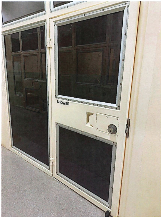
Figure 15 - Shower door at the Palmerston Watch House.
