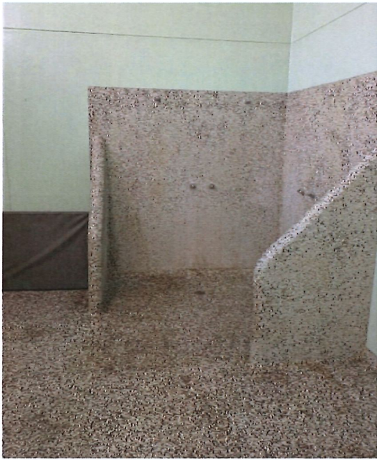
Figure 19 – Shower in the exercise yard at the Katherine watch house.
